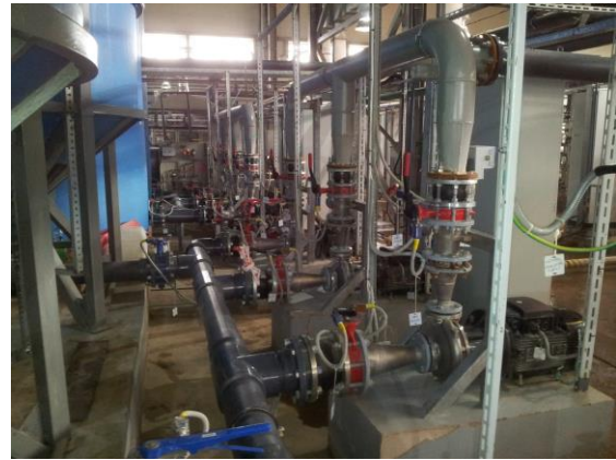
Photo: Industrial water recycling plant auditing in Amursk, The Russian Federation.
