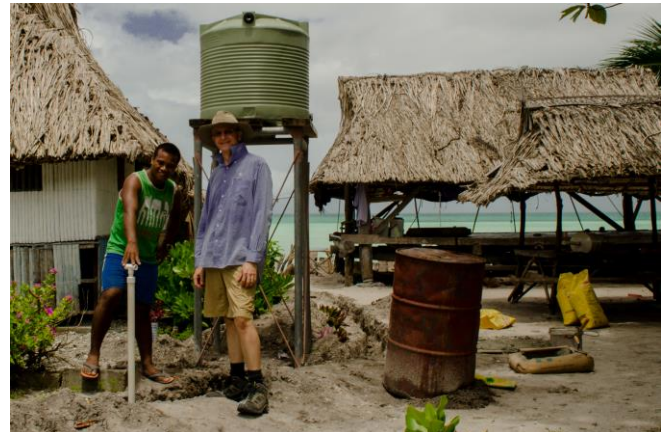
Photo: Village water supply installation on Abaiang Atoll, The Republic of Kiribati.
